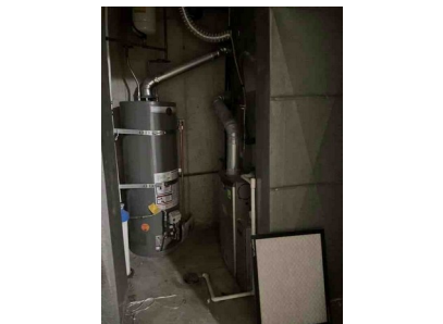
Mechanical (water heater and furnace)
